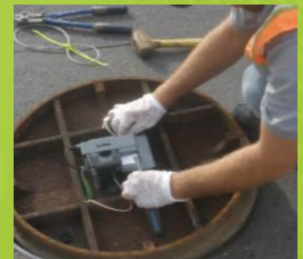
(Above) A Hadronex device installation in Anaheim.
